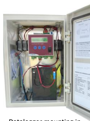
Datalogger mounting in the IP65 container
