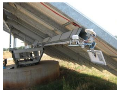
Meteorological sensors directly applied on the solar tracker
