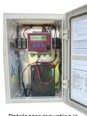
Datalogger mounting in the IP65 container
