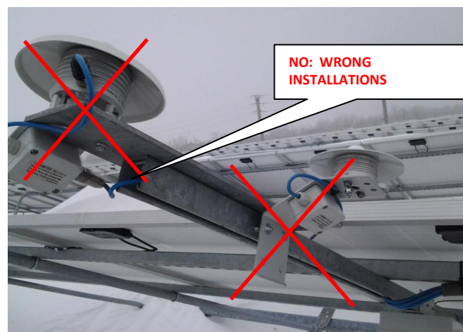
Picture 3 – Wrong installations
