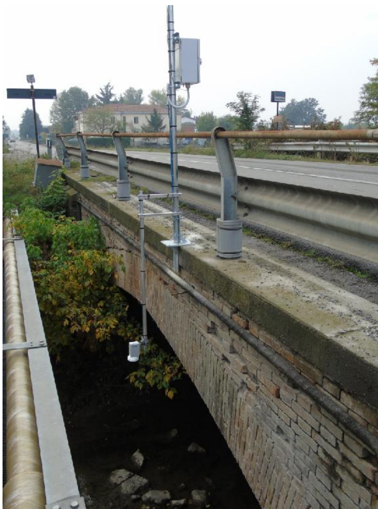
Picture 1 – Example of hydrometric station with sonic water level sensor
